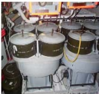
Figure 1: CDAUs in the fwd escape compartment of a SSN. Each CDAU holds 4 canisters.
